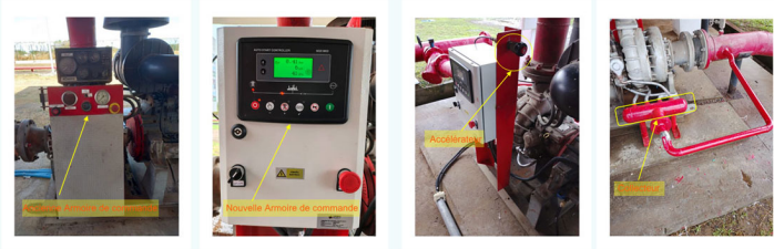
Manifold, old and new DCI motor pump group controls.
